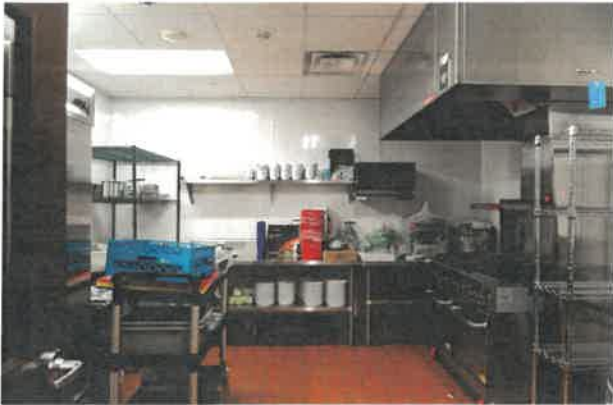
Finished commercial kitchen
